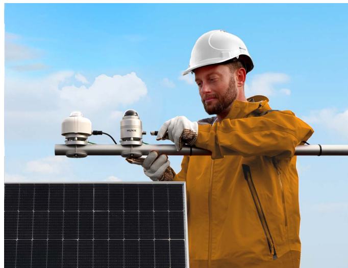
Figure 4 Typical installation of SRD100, next to a normal Class A pyranometer, such as the SR300-D1.
