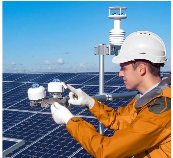
Figure 3 Two SR300 Class A pyranometers with digital output for GHI (Global Horizontal Irradiance) and POA (Plane of Array) measurement applications.
