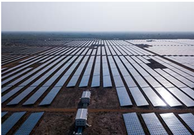
Figure 7 The Khavda PV power plant.
