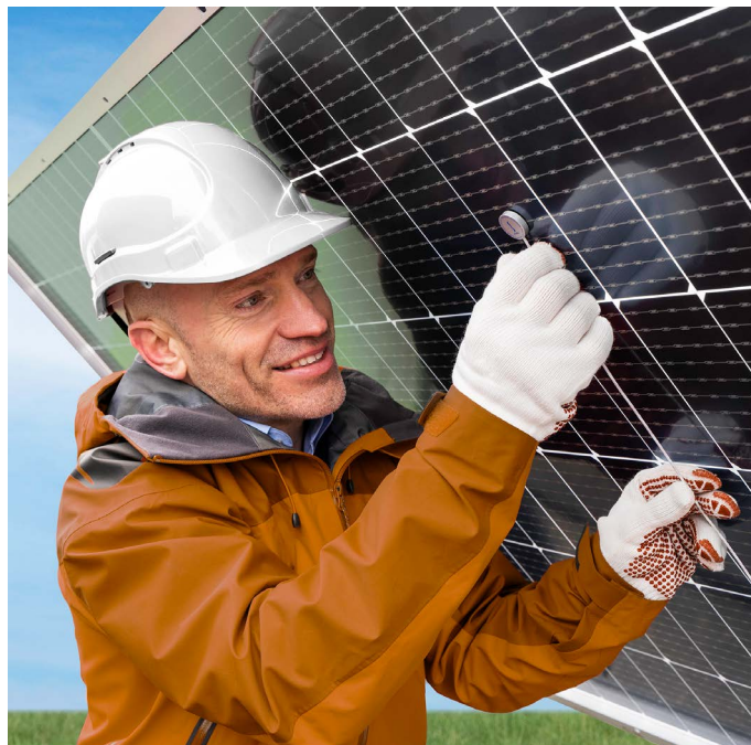
Figure 4 PVMT01 installed on the rear side of a PV module. The sensors are preferably installed at the center of a cell, close to the center of the module. IEC requires 3 sensors per monitoring station.
