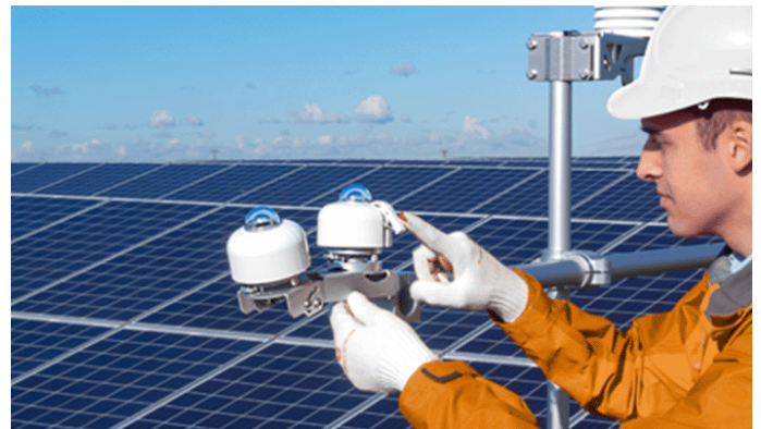
Figure 3 Two SR300 spectrally flat Class A pyranometers measuring GHI (global horizontal irradiance) and POA (Plane of Array) in a PV performance monitoring system.
