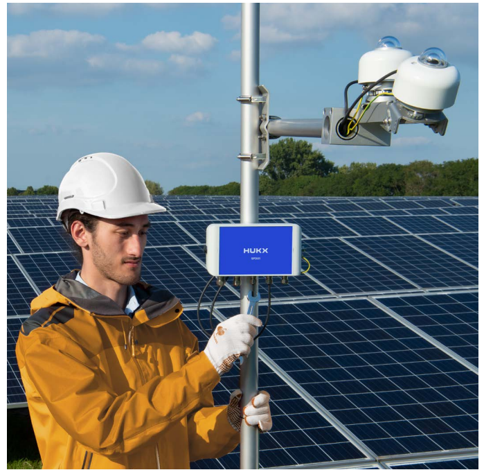
Figure 6 Two SR300-D1 pyranometers that are connected to the SPD01 Surge Protection Device. With the optional SPD01, you can upgrade surge immunity to level 4.
