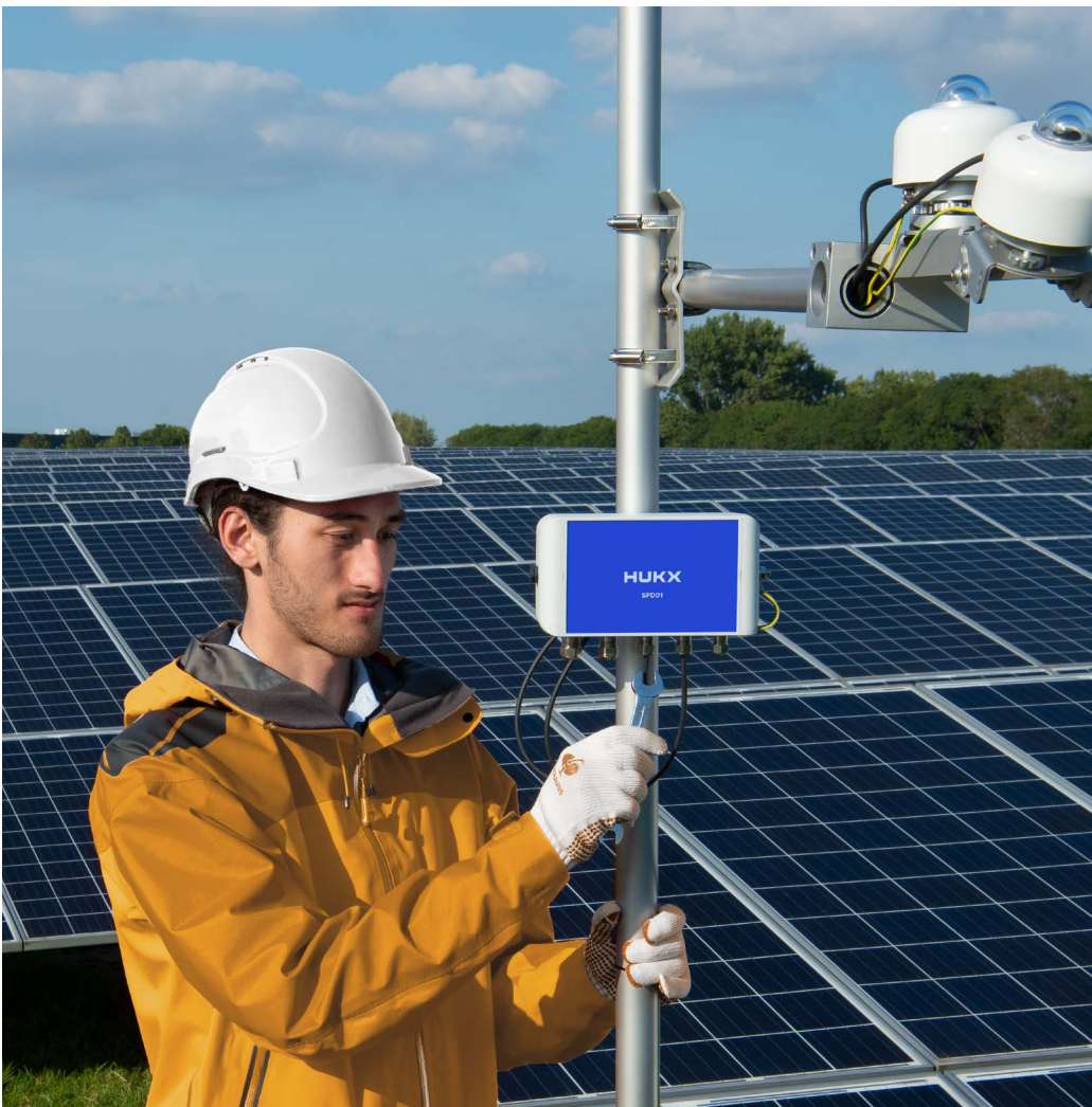
Figure 2 Surge protection upgraded to level 4. One SPD 1 Surge Protection Device can protect up to three instruments.
